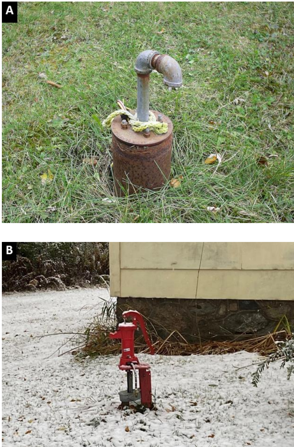
Figure 12. Panel A, LA-537 before initial visit for this grant period showing poor access due to compression fitting with original pump discharge plumbing. Panel B, further modifications on LA-537, making it inaccessible. Photos courtesy of U.S. Geological Survey.
