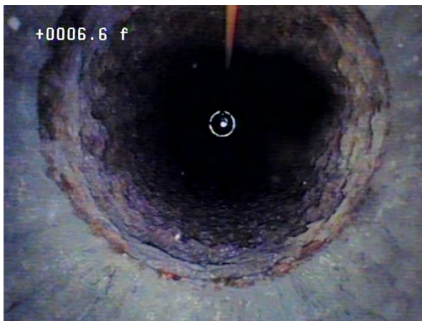
Figure 49. Screenshot from borehole video log collected October 26, 2021 on KE-46. Down-hole view of interval where casing condition changes from the smooth and relatively rust-free casing extension added in 1962, to the heavily rusted, lumpy and pitted original casing at approximately 7 ft BTOC. The bull's-eye like feature is camera lights reflecting off the water surface. Footage on image is in depth below top of casing as recorded by the video logging equipment.
