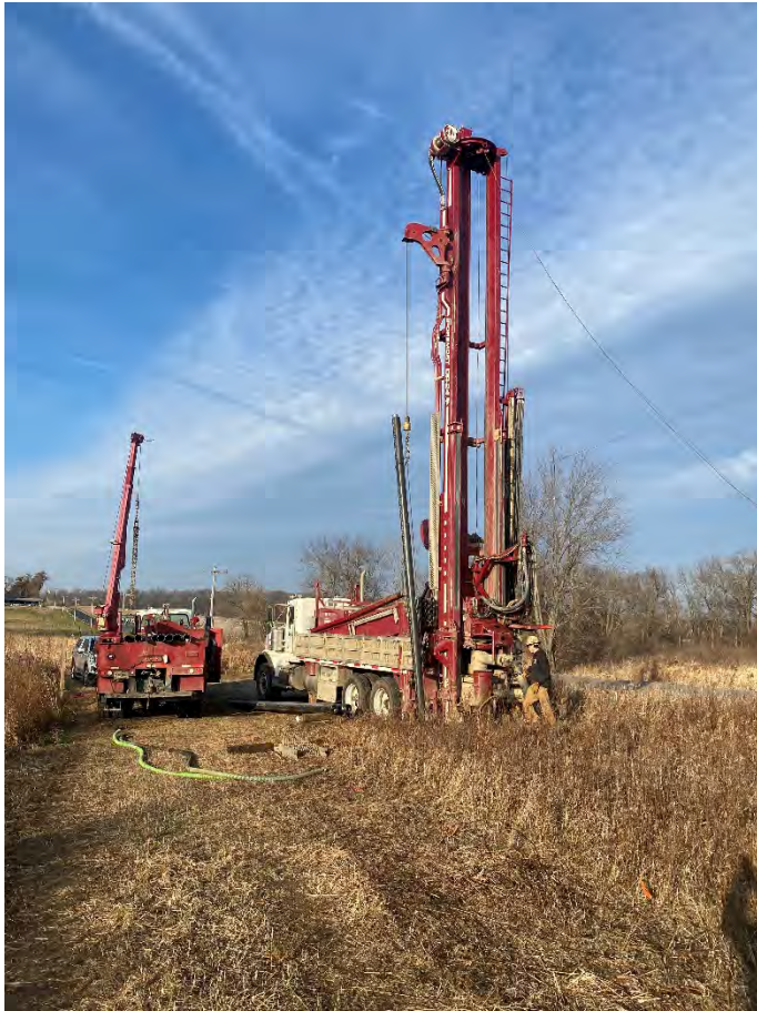
Figure 63. Sam's Well Drilling Inc. installed RO-1180 on December 10, 2021.
