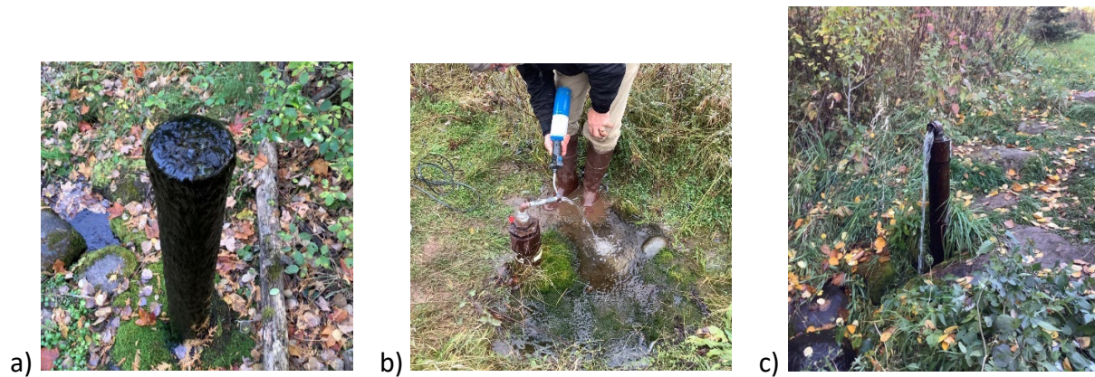
Figure 10. Examples of a) uncontrolled discharge of water from within the well casing (BA-FW-49), b) uncontrolled discharge and flooding in the vicinity of a flowing well (BA-FW-06), and c) uncontrolled discharge and surface erosion in the vicinity of a flowing well (BA-FW-20).
